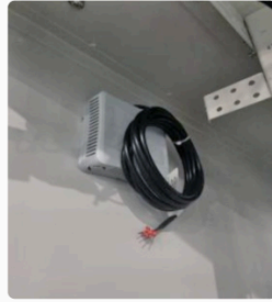
Temperature and humidity sensor
