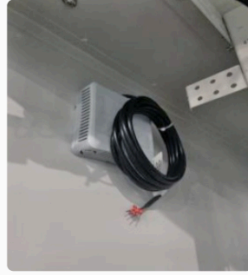
Temperature and humidity sensor
