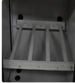
Battery bearing rack
