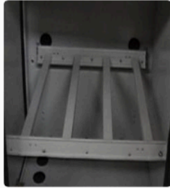
Battery bearing rack
