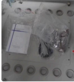
Cable entry holes
