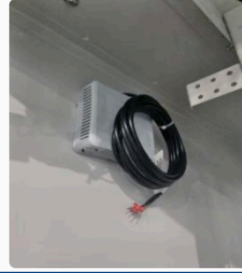
Temperature and humidity sensor
