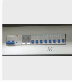
AC power distribution box
