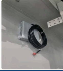
Temperature and humidity sensor
