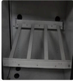
Battery bearing rack
